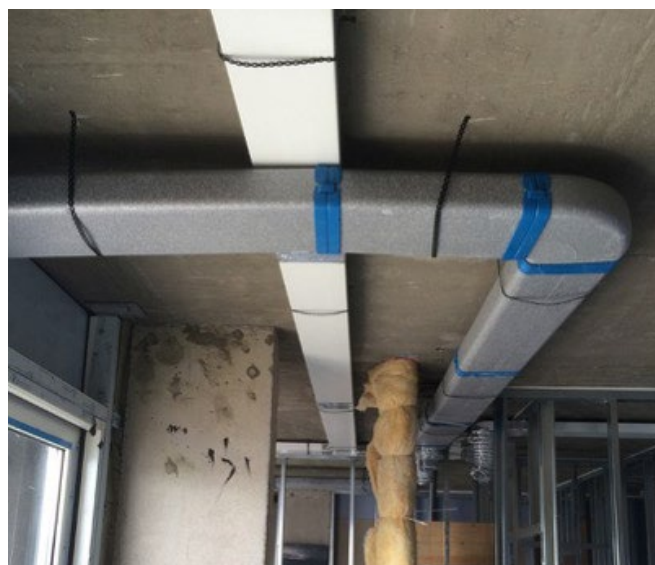
Ducting at Site 2 – Rigid duct installation. Straight duct runs using proprietary bends where needed. Intake/exhaust ductwork is pre-insulated (grey ducting). Ducting mechanically connected and fastened throughout
