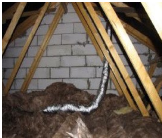
Ducting at Site 3 – Long looping ducting could cause condensation to build up and increase the required fan power
