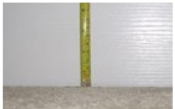
Site 1 – Example of inadequate door undercut
