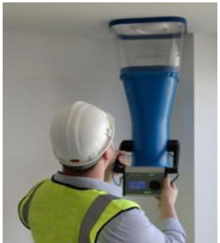
Measurements of air flow rates being made by a member of the Hub team using a powered automatic compensating volume flow meter
